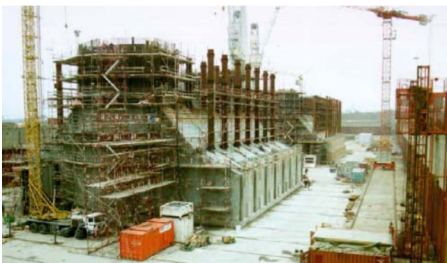
Fig. 7.9: Graving Dock Construction of Concrete Bridge Pier Caissons for Oresund Crossing, EM1110-2-2611, C-8
