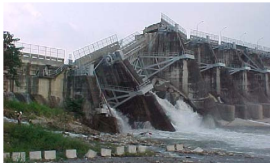
Fig. 5.9(b): Collapse of a weir due to foundation failure.
